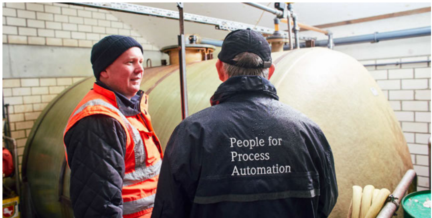
Precipitant tank at Stadtlahn WWTP: An iron(III) chloride ( \text{FeCl}_3 ) precipitant is used in summer, while an iron-aluminum combination product is used in the winter months.
