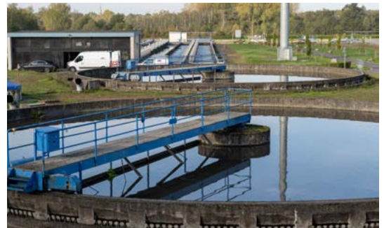
Wastewater treatment plant in Wasmuël in Belgium
