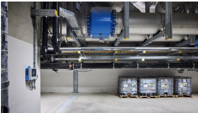
Proline Promag W 400 DN 700 flowmeters measure the volume flow of the purified water on its way to the Rhine.
