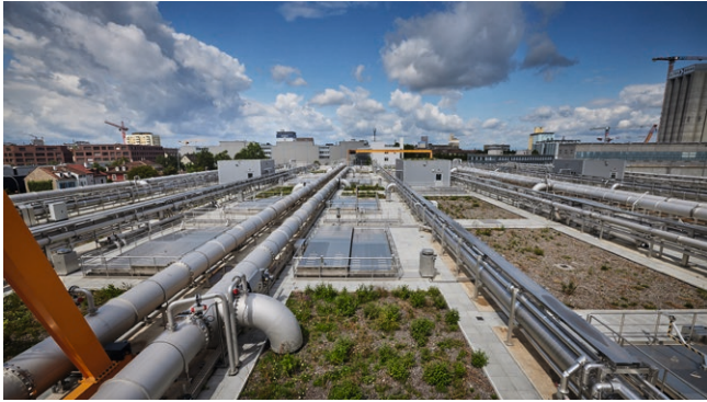
View of the sequence batch reactors at the ARA Basel wastewater treatment plant.
