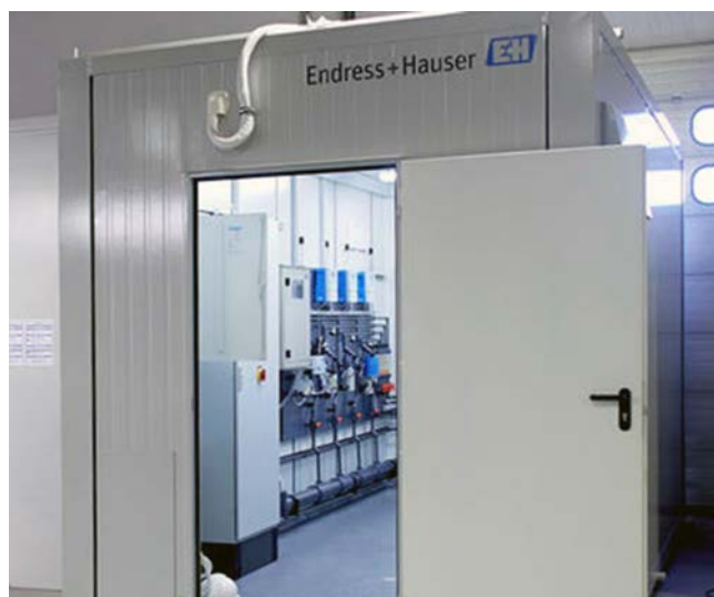
Endress+Hauser analytical instruments and sampling components user-friendly mounted in an air-conditioned shelter
